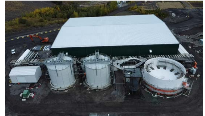
Image: The six-million-litre-per-day MBBR water treatment facility at Brule Mine
