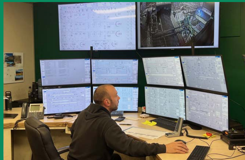
Image: Quintette processing plant control room
