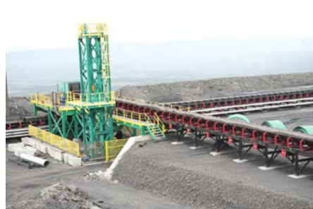
Image: Quintette Overland Conveyor
