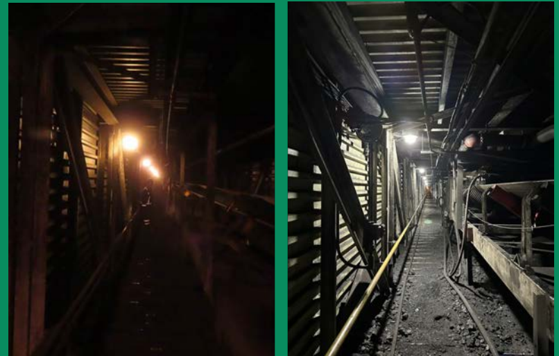
Image: Before (left) and after (right) photos of energy efficient lighting upgrades at Quintette
